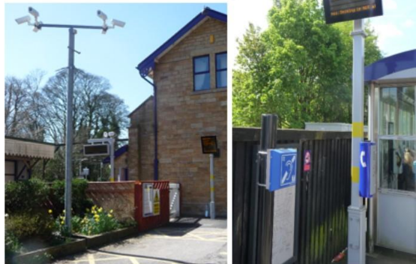
Examples of equipment installed under the Rail Station Improvement Strategy – CCTV, Customer Information Screens, Help Points, Induction Loops
